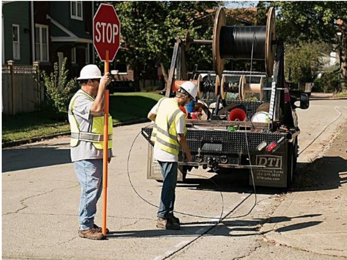
Figure 2 It took only 5 months for Google to lay its fiber in Louisville, KY, mostly using microtrenching. (Source: Tech Republic)
